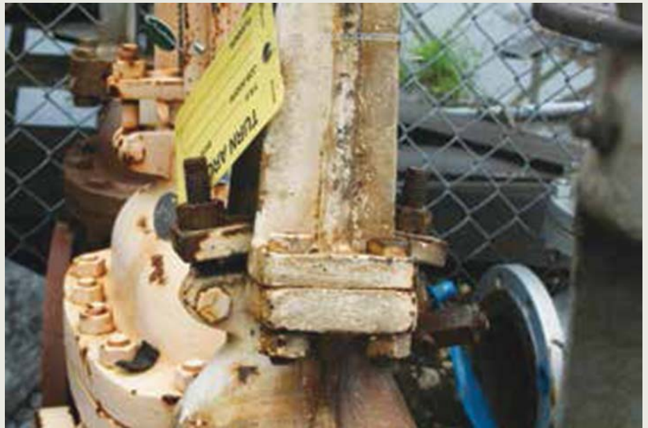
Image 2. An example of a valve that should be replaced.
